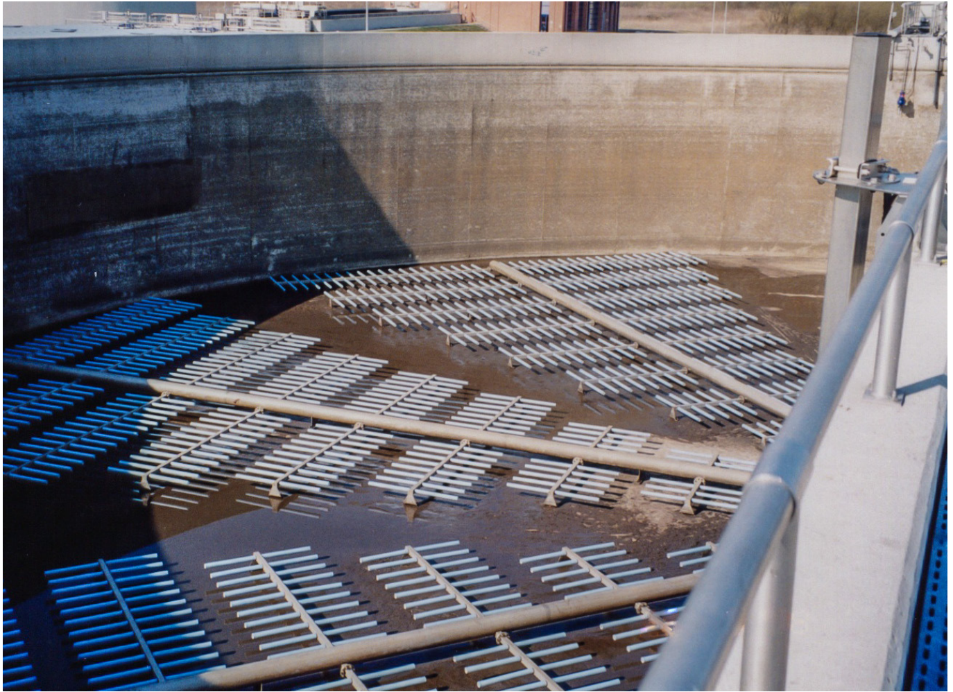
BUTTING pipes for better quality of life – here in a water treatment plant
