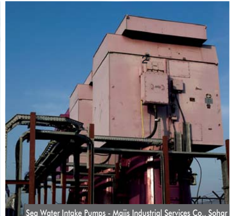
Sea Water Intake Pumps - Majis Industrial Services Co., Sohar
