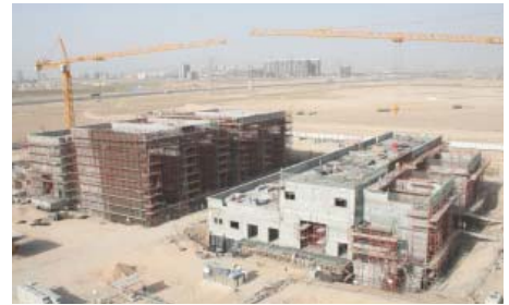
DubaiLand-2 Sub-station Project for DEWA/Siemens
